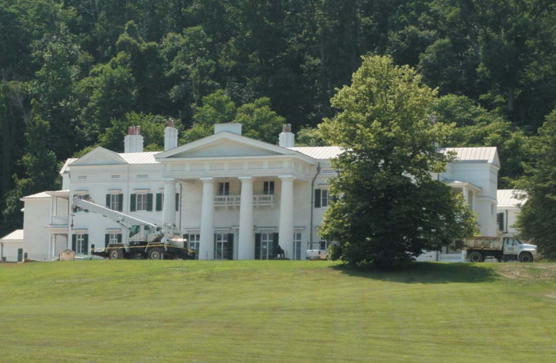
Built in 1750 and extensively remodeled in 1870, Morven Park is closed for renovations and should reopen by April 2009.
