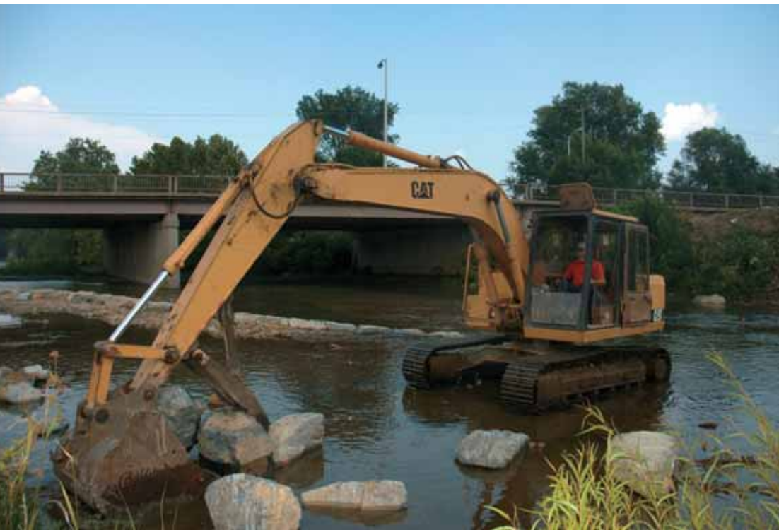
Heavy equipment was used on the South River to help improve habitat for the river's fish.
