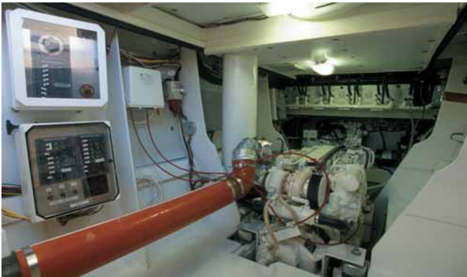
The large, spacious engine room allows plenty of space for inspection and maintenance.
